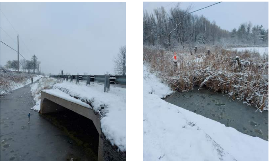
Existing conditions at Crossing 34 on the south side of Leitrim Road. Left photograph is facing southwest along the roadside ditch; right photograph is taken facing southeast towards downstream.
