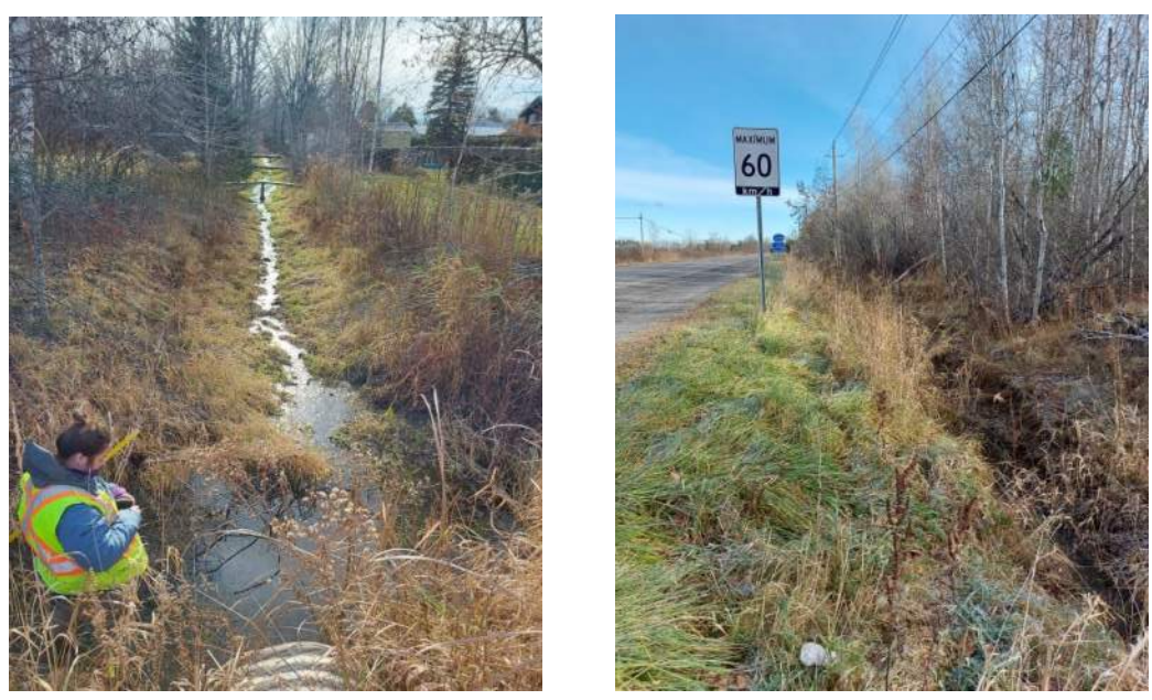
Existing conditions at Crossing 2 on the south side of Piperville Road. Left photo is facing southeast at a drainage ditch flowing into the culvert from properties south of Piperville Road; right photo is facing northeast at the roadside ditch.
