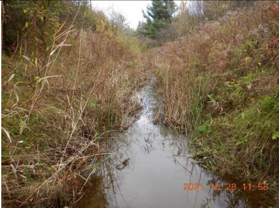
Reach backwatered due to large downstream beaver dam, instream logs and trees observed due to bank failure.
