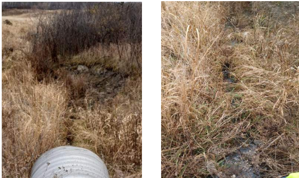
Existing conditions at Crossing 31 on the west side of Ramsayville Road. Left photo is taken facing west; right photo is taken facing downwards at the mouth of the culvert.
