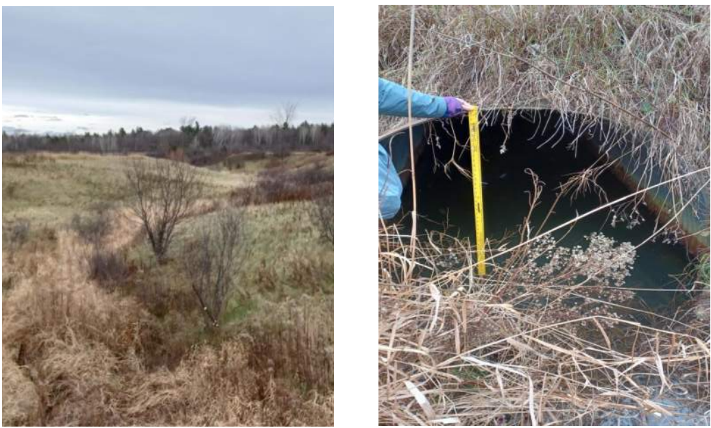
Existing conditions at Crossing 29 on the east side of Ramsayville Road. Left photo is facing east; right photo is facing west into the mouth of the culvert.
