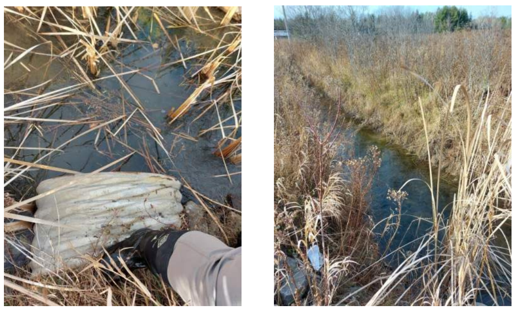
Existing conditions at Crossing 2 on the north side of Piperville Road. Left photo is facing down at the culvert opening; right photo is facing southwest at the roadside ditch towards Crossing 1.
