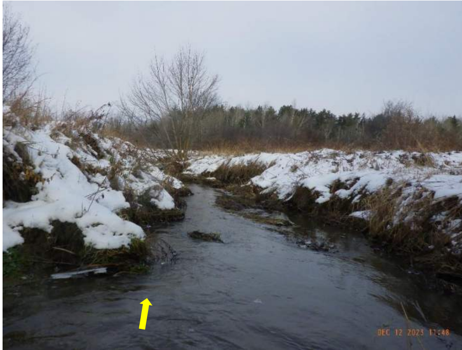
Channel meandered through agricultural fields. No riffle-pool formations. Slumping and undercutting was common.
