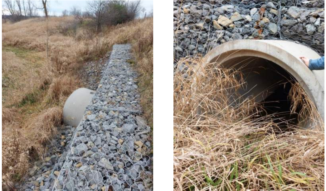
Existing conditions at Crossing 13 on the south side of Russell Road. Left photograph is facing northeast; right photograph is facing south towards the culvert.
