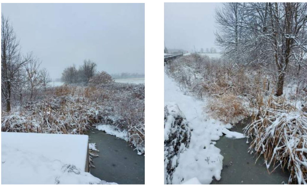
Existing conditions at Crossing 34 on the north side of Leitrim Road. Left photo is taken facing northwest; right photograph is taken facing west along Leitrim Road.
