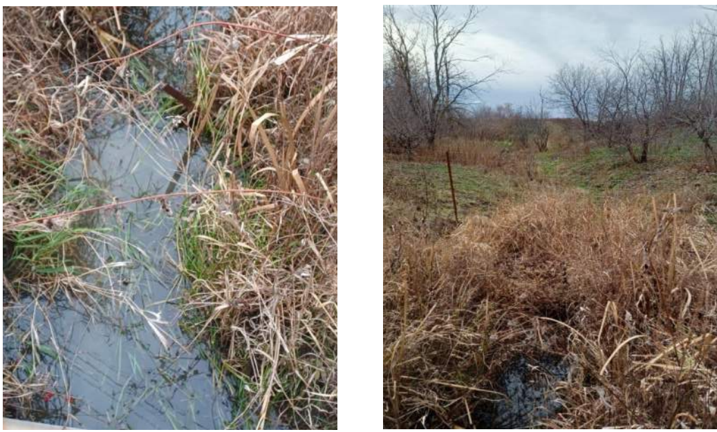
Existing conditions at Crossing 29 on the west side of Ramsayville Road. Left photo is facing down at the mouth of the culvert; right photo is facing west.
