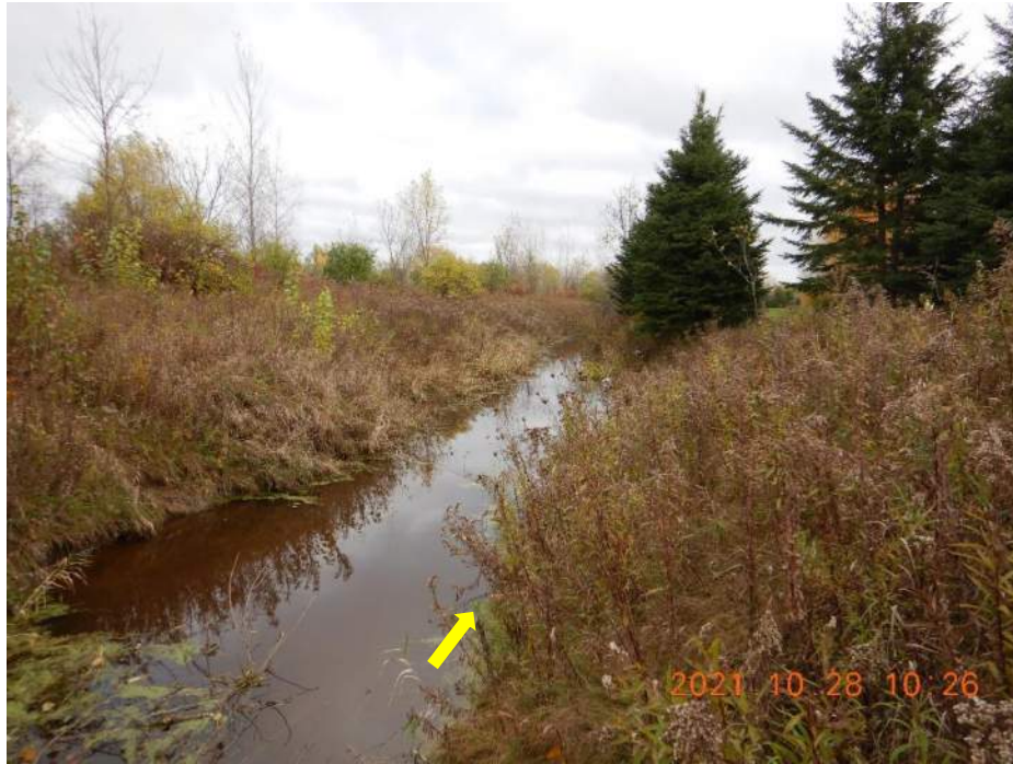
Evidence of enlarging, erosion and minor adjustment may be related to beaver activity
