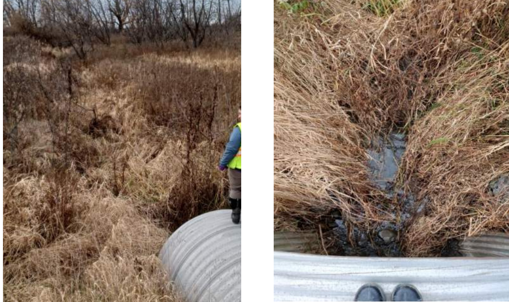
Existing conditions at Crossing 31 on the west side of Ramsayville Road. Left photograph is taken facing west, upstream; right photograph is taken facing down at the mouth of the culvert.
