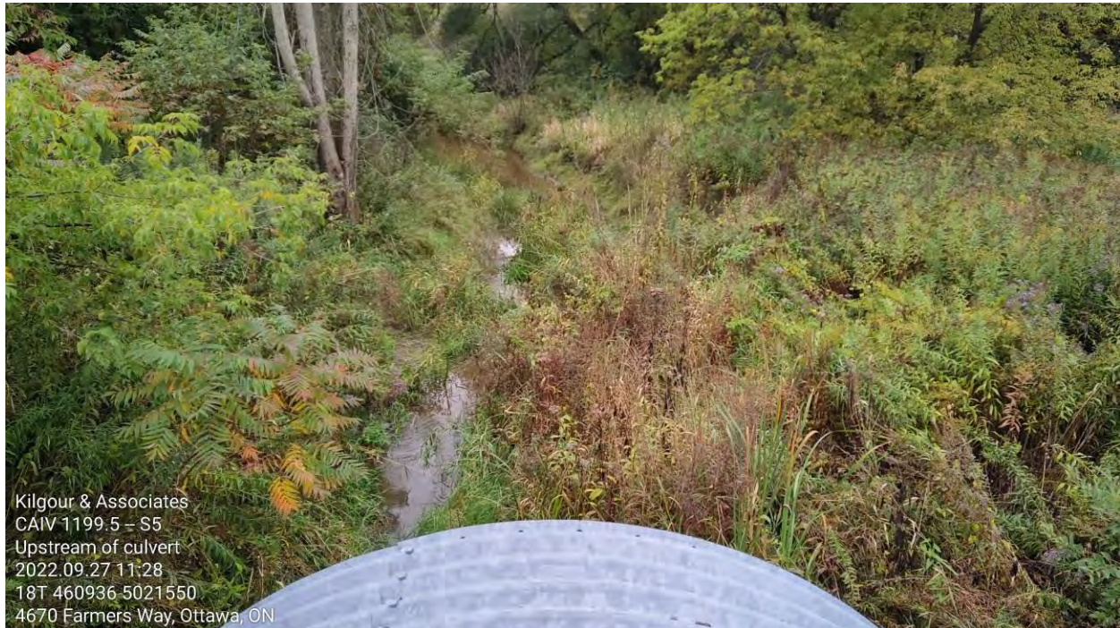
Figure 54 Upstream view of the culvert inlet at S5 (photo taken on September 27, 2022)
