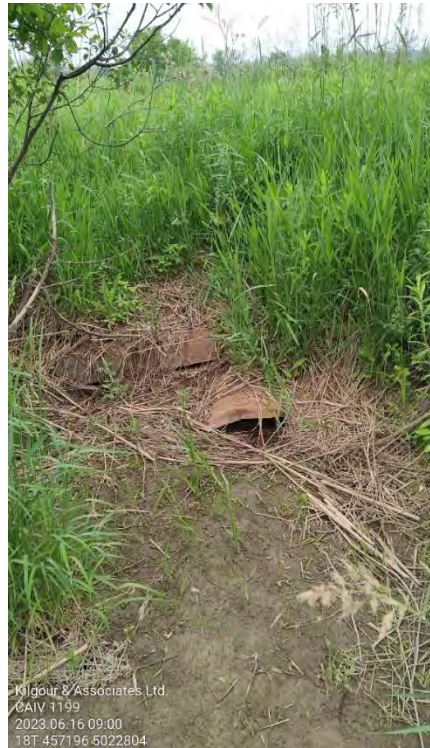
Figure 68 Picture of the culvert locate in the upstream section of the unnamed Ramsay Creek tributary surrounded by the agriculture field, June 16, 2023
