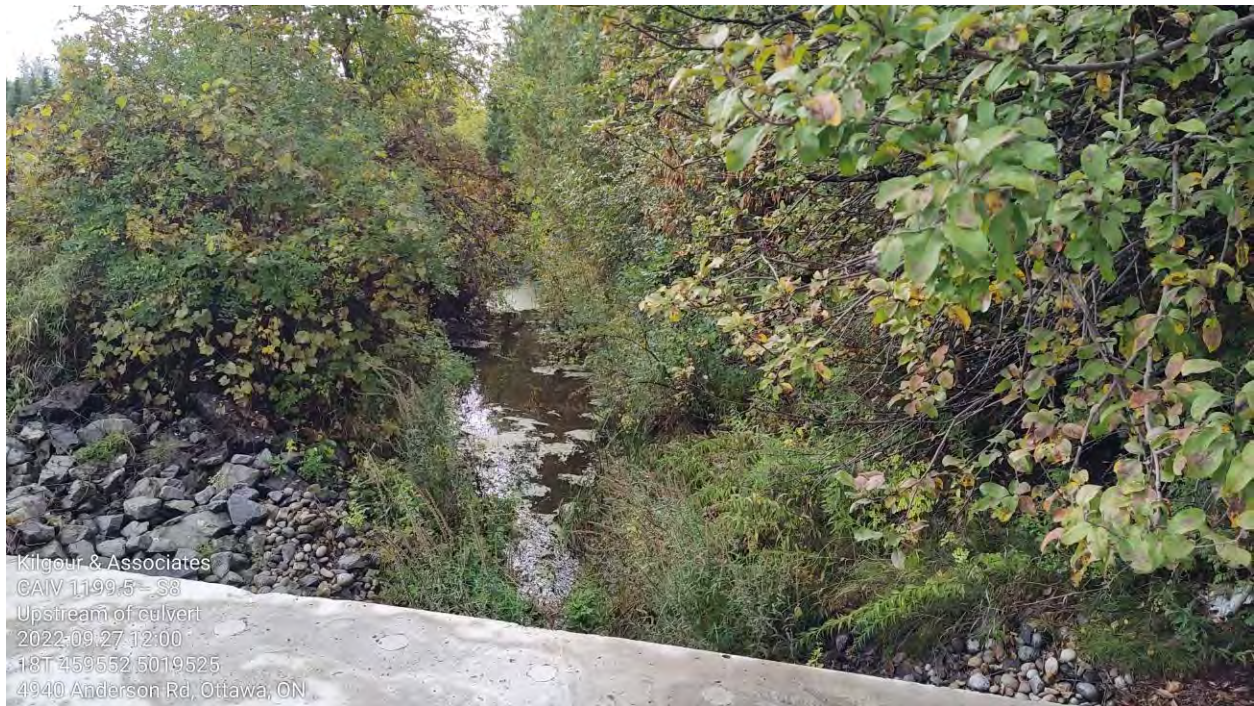
Figure 56 Upstream view of the culvert inlet at S8 (photo taken on September 27, 2022)
