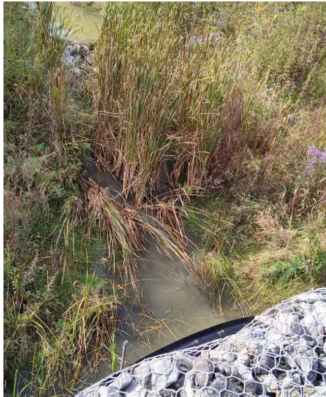
Figure 55 Upstream view of the culvert inlet at S6 (photo taken on September 27, 2022)
