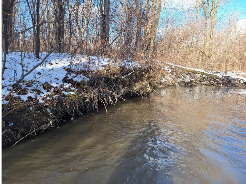
Undercutting and exposed roots was observed at several locations along the reach. The channel substrate was composed of fine silts over compact clay.
