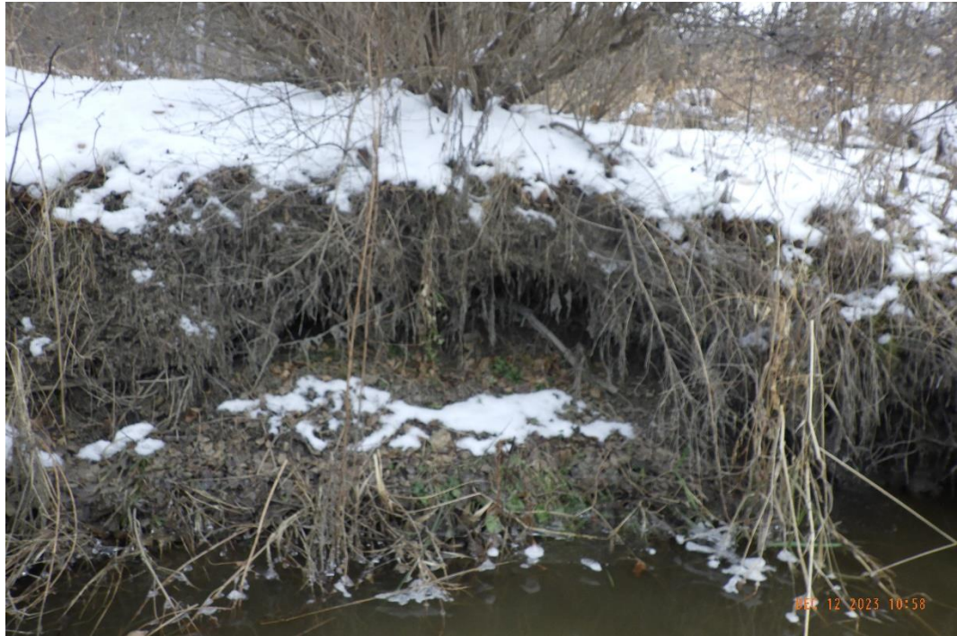
Slumping occurred in localized areas along the reach primarily in the downstream portion. Basal scour was also observed through more than 50% of the reach.
