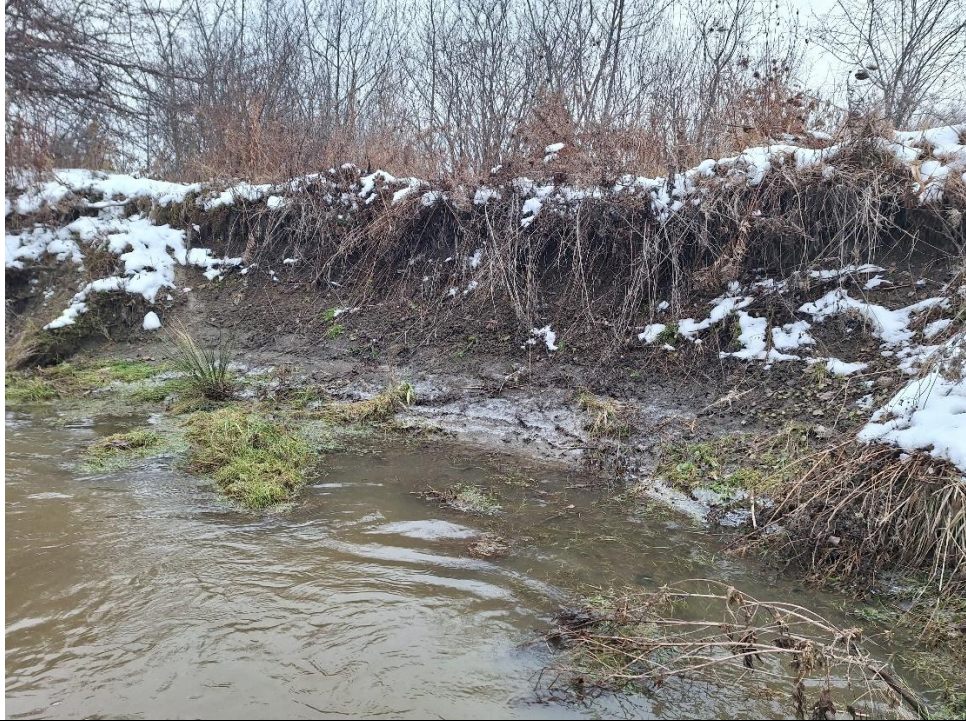
Basal scour and undercutting were observed throughout more than 50% of the reach with scour occurring along the inside of meander bends and through the riffles.
