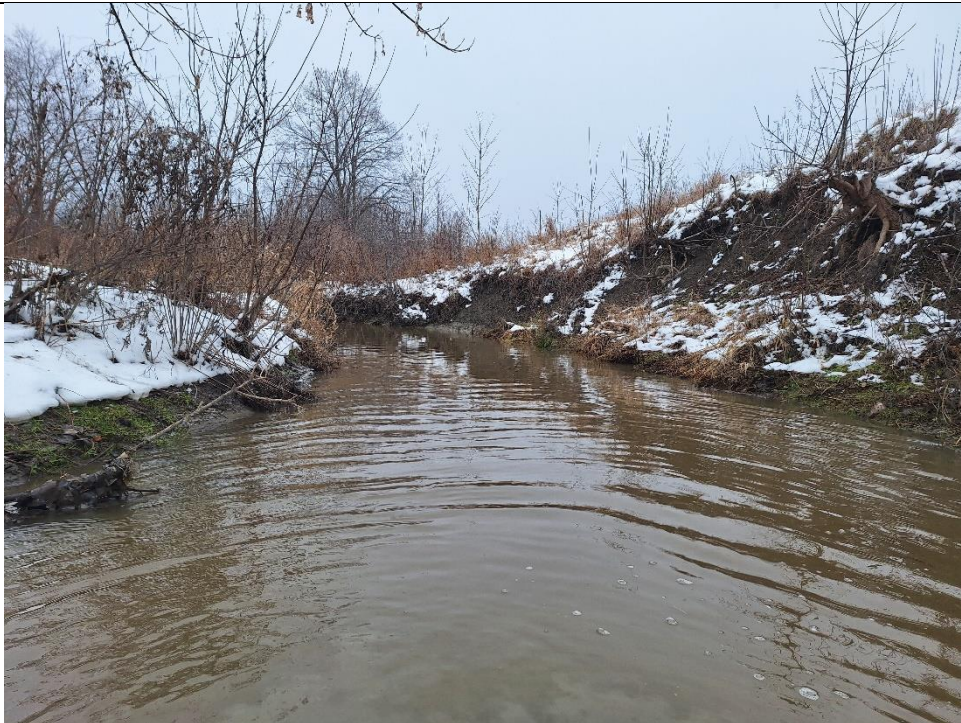
The channel bank was observed to be eroding adjacent to the train tracks.
