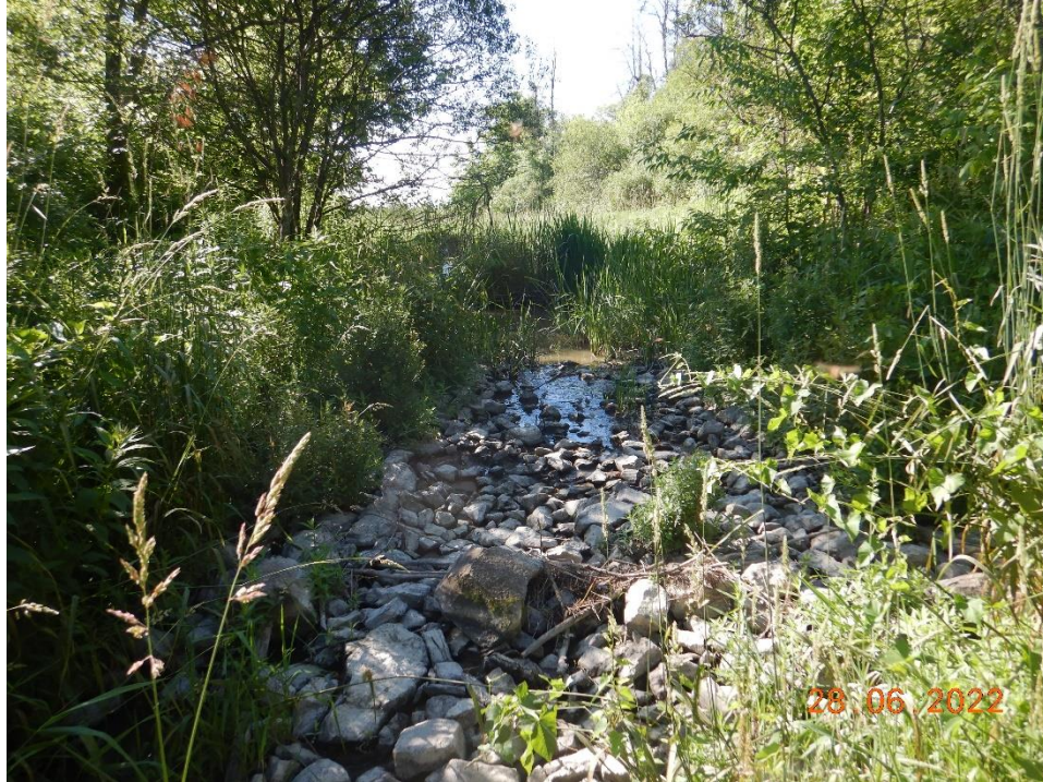
Placed cobbles were observed halfway through the reach. This caused a back water effect upstream, where the channel is wide a flat.
