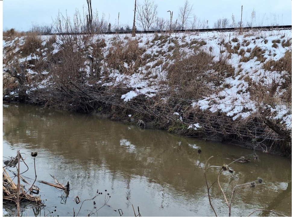
Undermined fencing was observed along the reach due to erosion and basal scour. Basal scour and undercutting was observed commonly throughout the reach.
