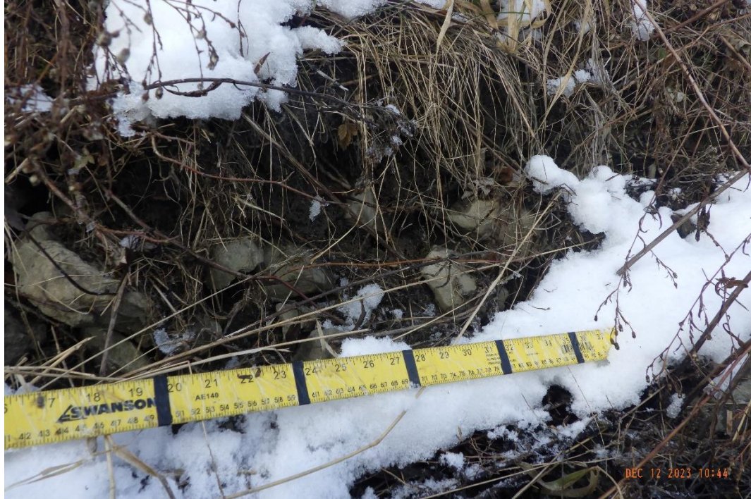
A significant armour layer was identified to be suspended within the banks.
