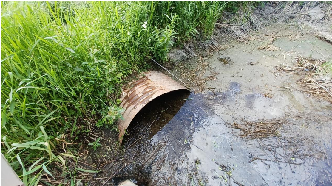
A historic farm crossing was observed along the upstream extent of the reach. The buried culvert has caused backwatering.
