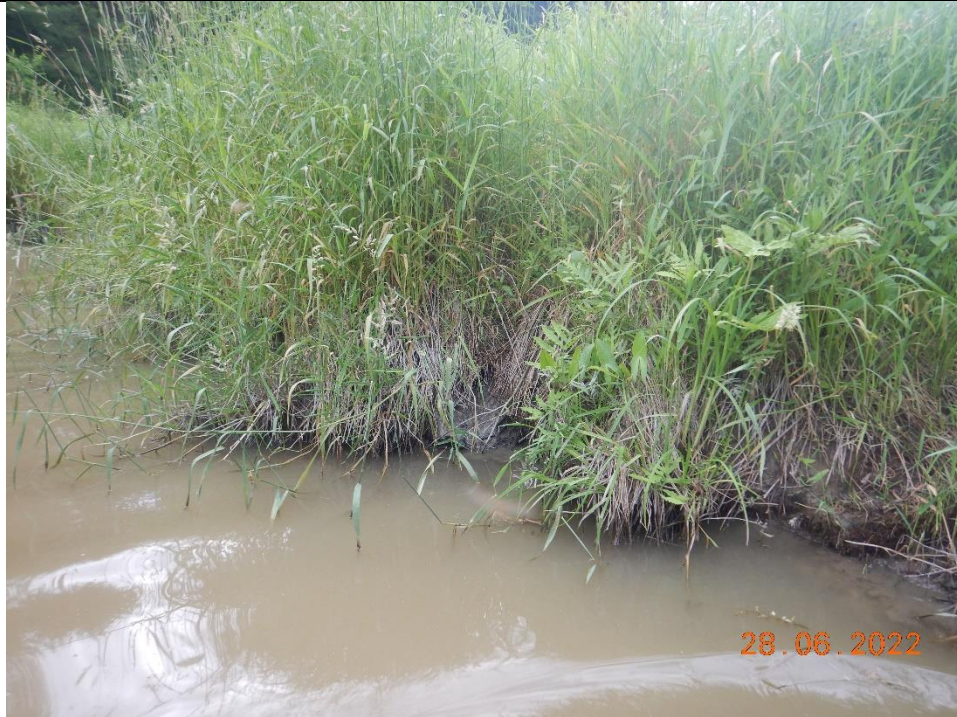
Slumping was commonly observed throughout the banks on both sides of the channel.
